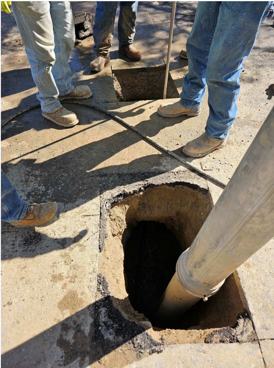
Emergency leak that came in late in the day.
