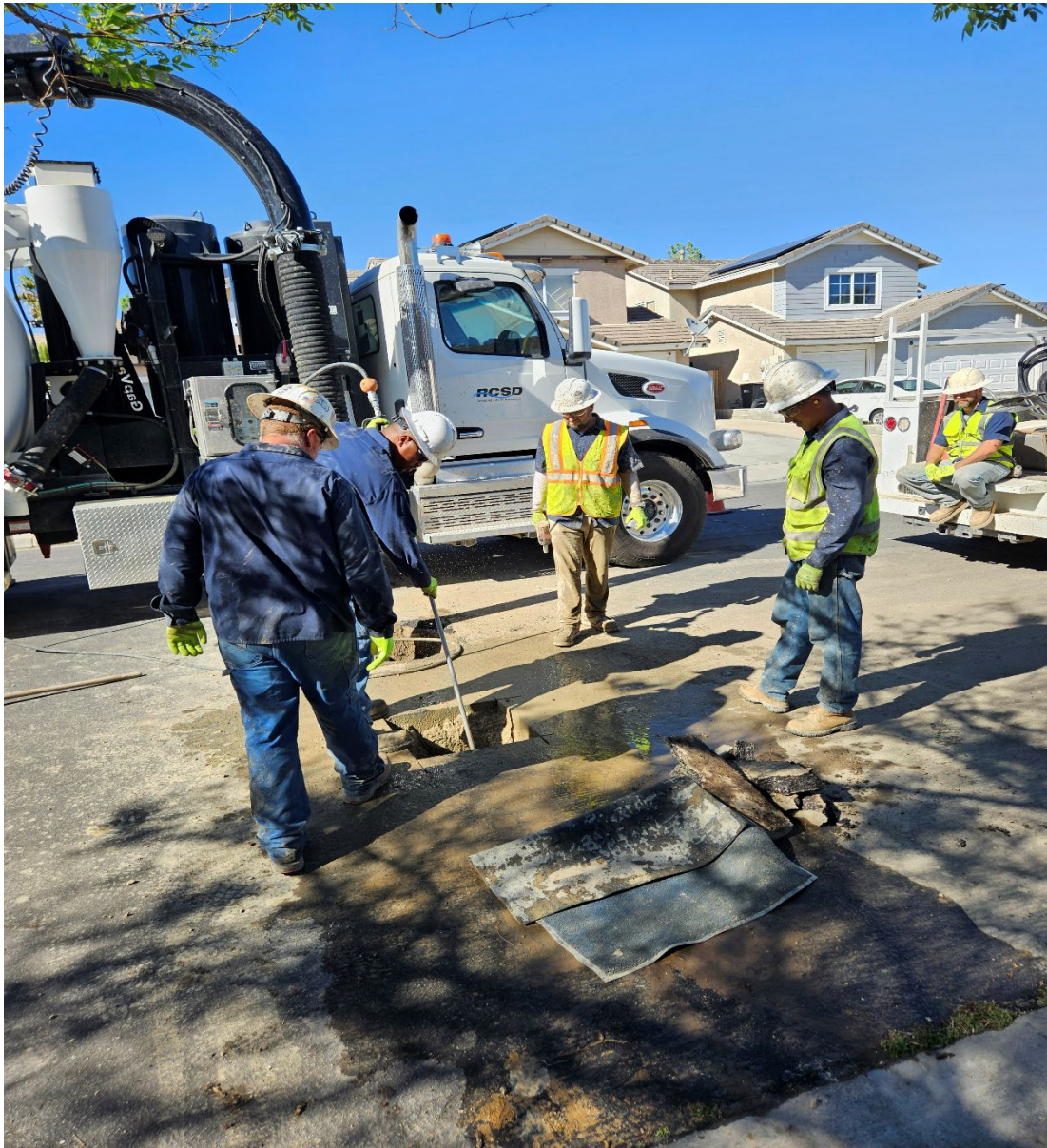
Emergency leak being located with hydro excavation.
